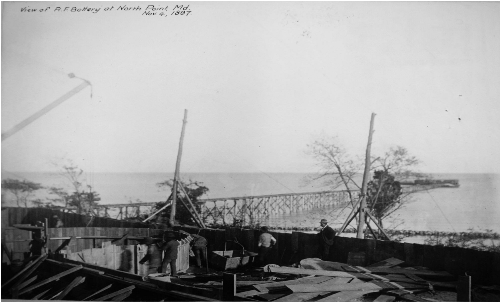
Battery Harris being constructed in 1897. Note the long construction pier. A small locomotive pulled cars full of building materials along the pier into the construction sites.
