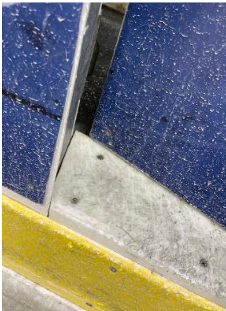
#7 Bent door hitting poly threshold.
