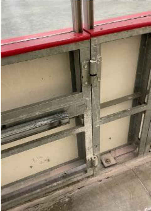
#13 Equipment Gate hinges not installed correctly.
