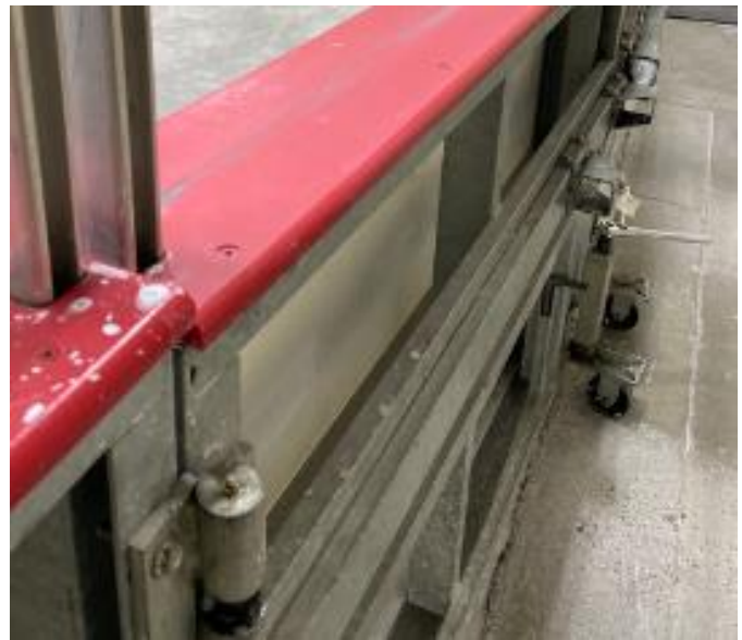
#14 Equipment gate casters are failing.
