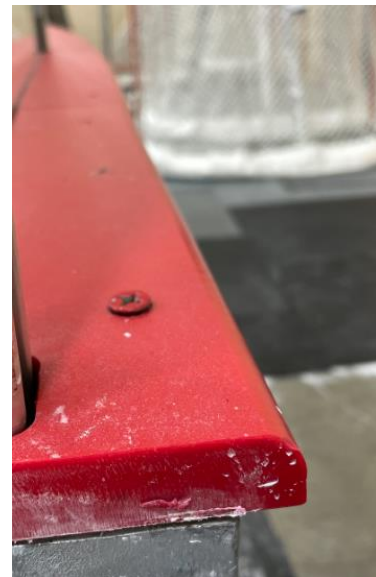
#35 Loose cap rail fasteners.
