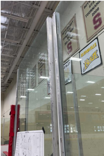
#20 Termination Shielding Supports not aligned
