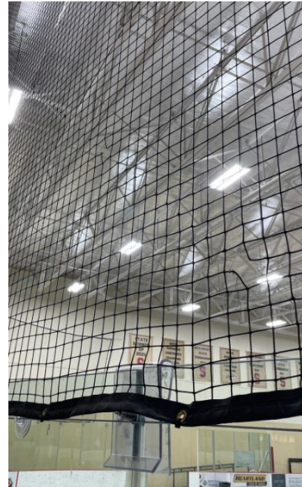
#33 3 Holes in netting lobby end.
