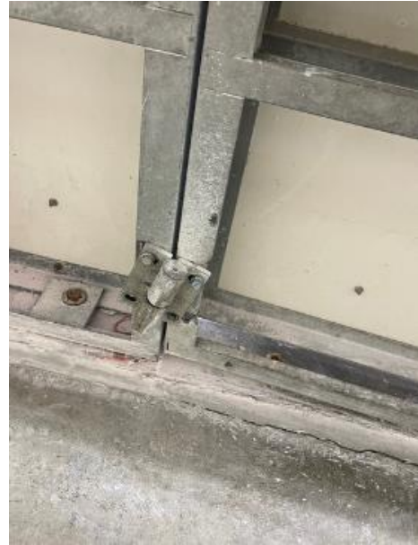
#10 Equipment gate hardware failing.
