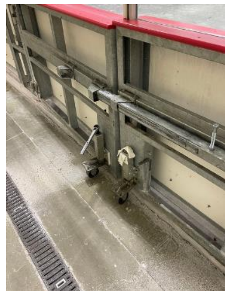
#12 Equipment gate slide bar not aligned.
