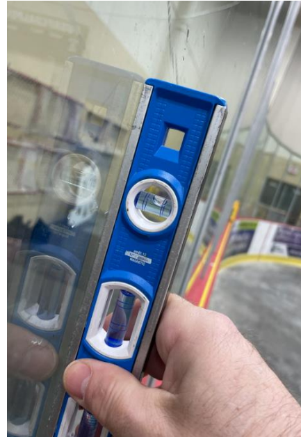
#2 Glass leaning into rink.
