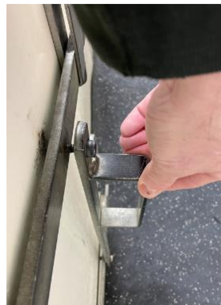
#8 Loose gate fasteners (All Gates)
