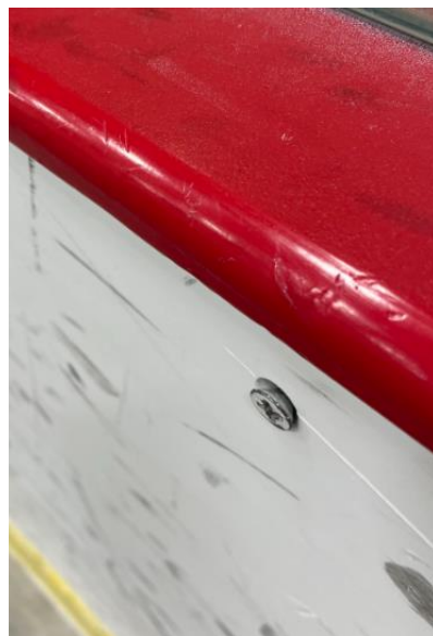
#30 Loose fasteners in multiple locations.
