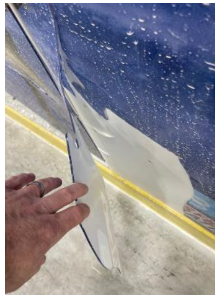
#4 Broken Lexan at gate door panel.
