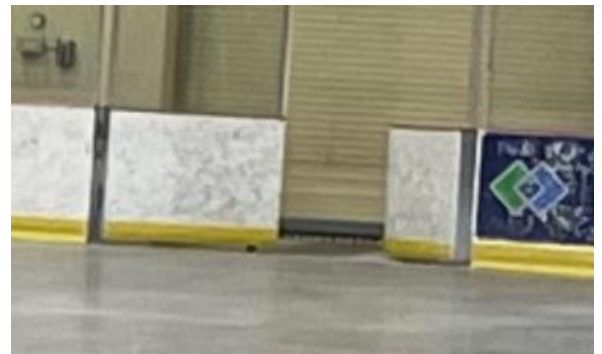
#31 Missing EQ Threshold
